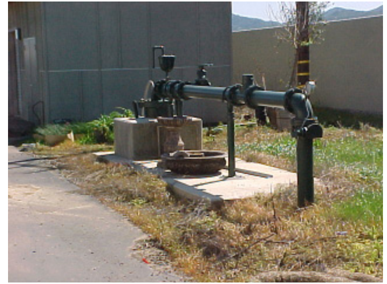
A Ground Water System Well
