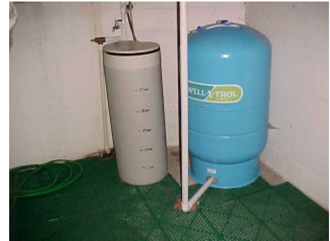
A Hydropneumatic Storage Tank
